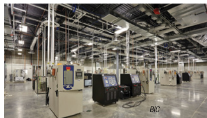
FIGURE 1. The Battery Innovation Center, located in Indiana, conducts research, development and testing of energy-storage systems
